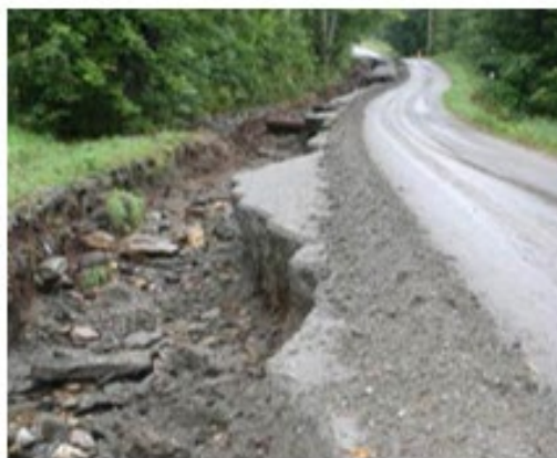
Gully Erosion = depth of 12" +
