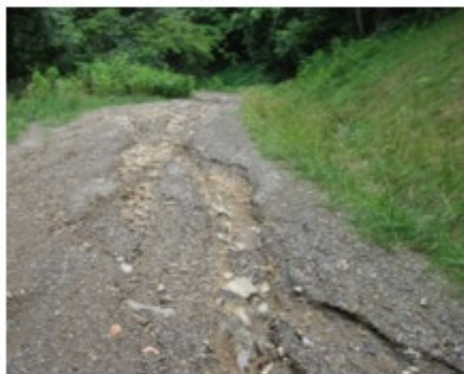
Rill Erosion = depth of 1" < 12"
